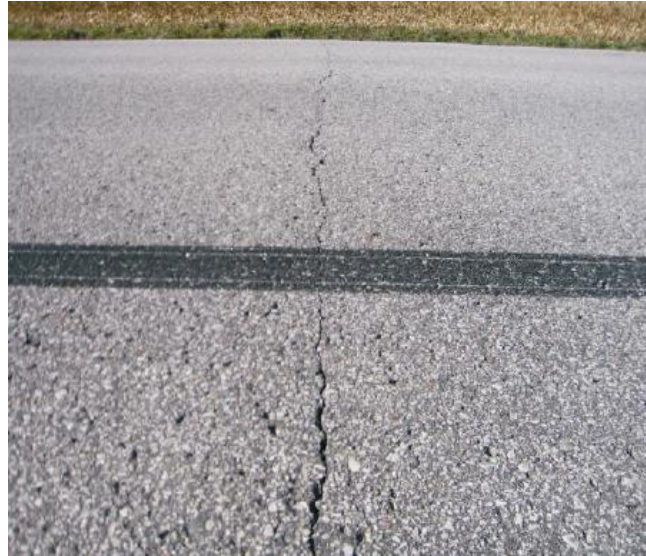
Low temperature cracking
