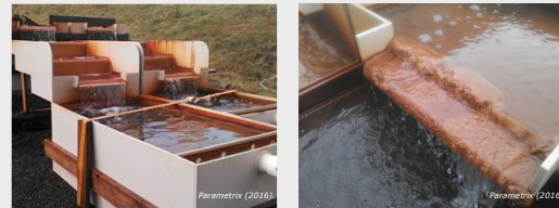
Image 3. Parametrix pilot study of cascade aeration, polymer flocculation, and settling experienced excess clogging and build-up from the iron precipitate.
