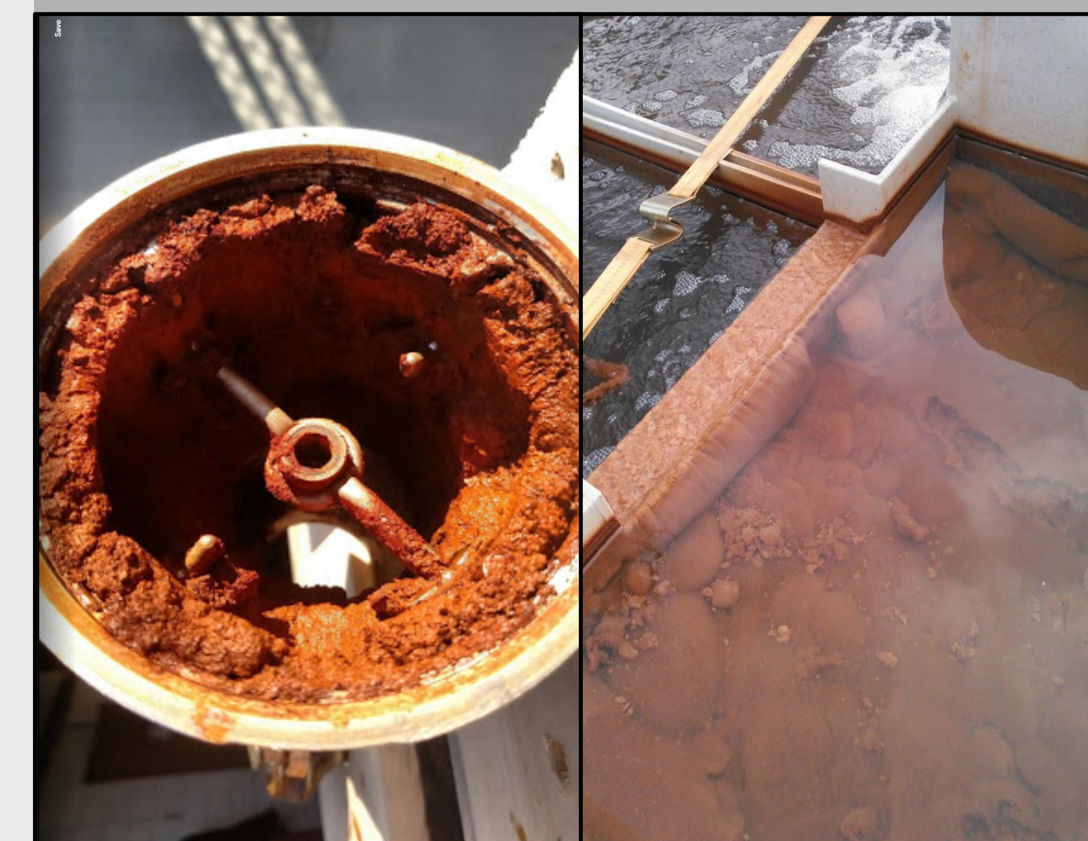
Figure 4. Iron build up inside of previously tested treatment system.
