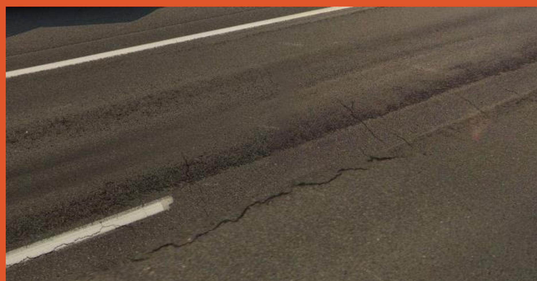
EXISTING PAVEMENT CONDITIONS
